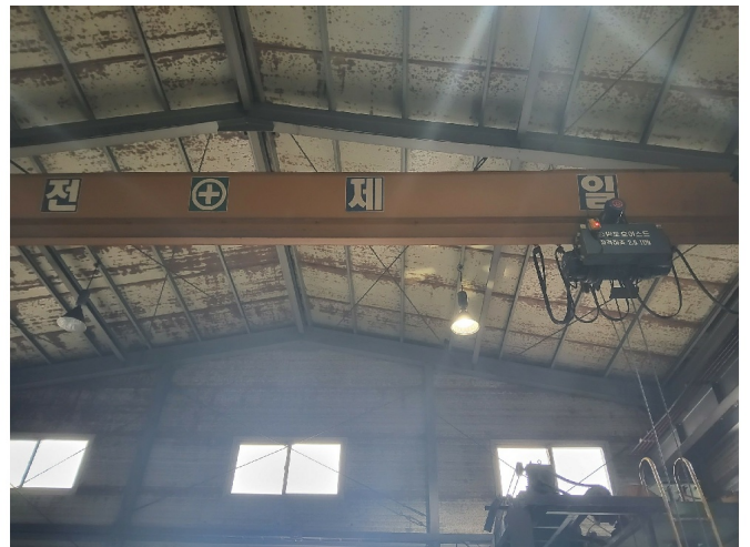
(2): Over Head Crane
