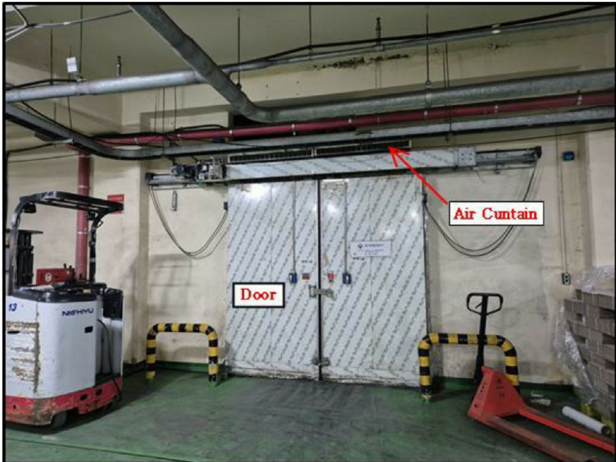
[ 1-(1)-1 , Door, Air Cuntain ]
